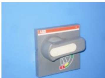
Picture 4-4: Circuit switch
