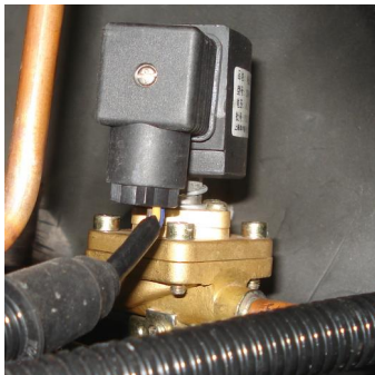
Picture 2-8: Hot Air Bypass Valve
