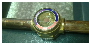
Picture 2-11: Refrigerant Indicator
