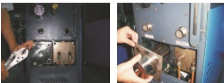
Picture 6-8: Pipe Heater 3
