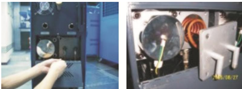
Picture 6-10: Cooling Pipes 2
