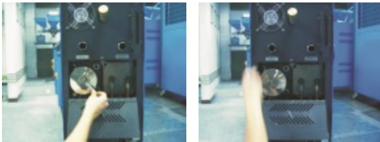
Picture 6-7: Pipe Heater 2
