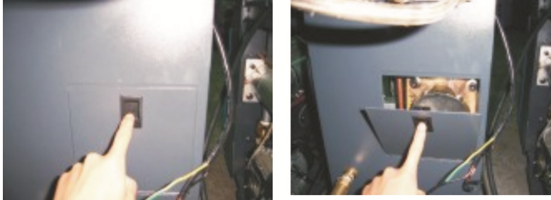
Picture 6-6: Pipe Heater 1
