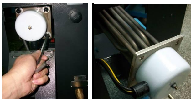
Picture 6-7: Pipe Heater 2
